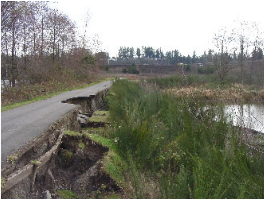
Figure17–Site d, Figure13–East-to-west view of embankment failure (lateral spread) at Capitol Interpretive Center (Photo from Bray and others, 2001). (GPS location: N47.02447°, W122.90784°).
