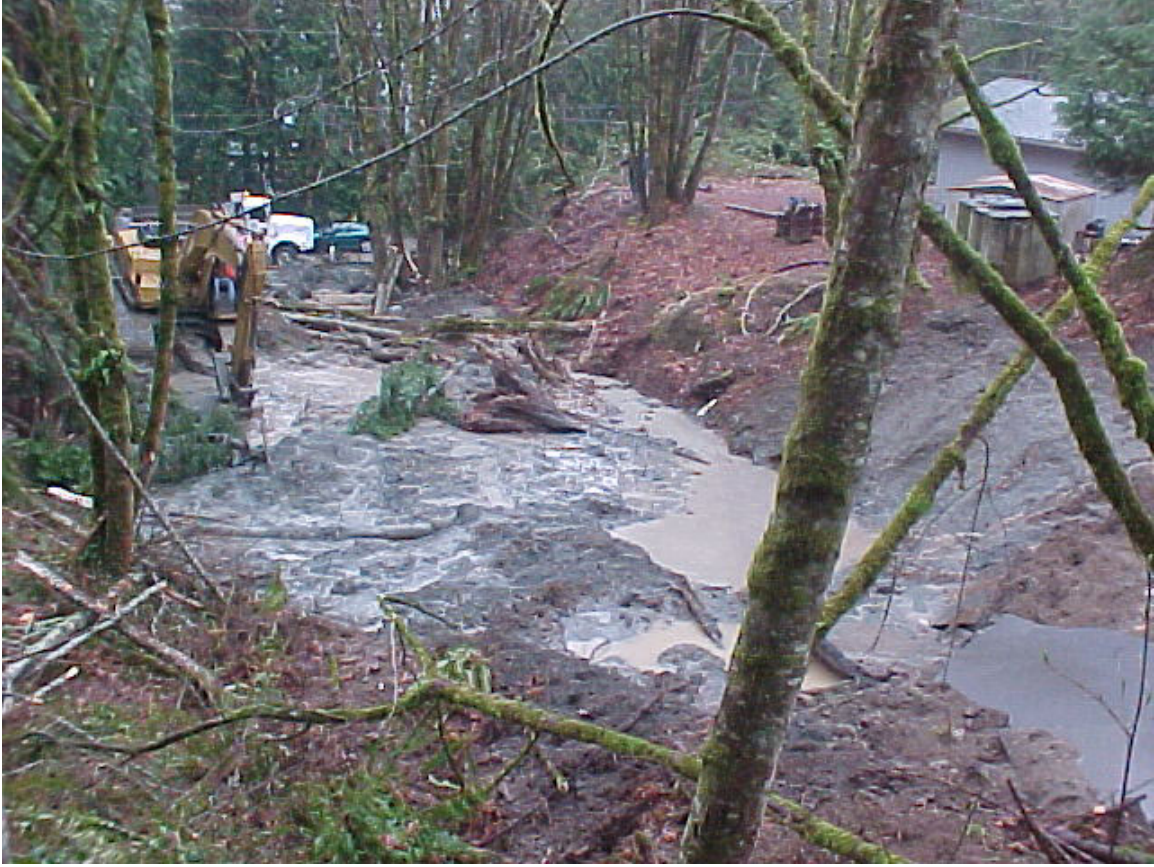
Figure 23.--View of runout of material down slope from the U.S. Highway 101 earth embankment landslide (Photo from Bray and others, 2001) (GPS location: N47.05834°, W123.01365°).
