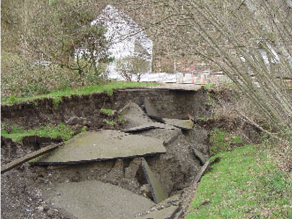
Figure 18–Site e, Figure 13–Failure of embankment due to liquefaction and lateral spreading at Capitol Interpretive Center (Photo from Bray and others, 2001). (GPS location: N47.02525°, W122.91000°).
