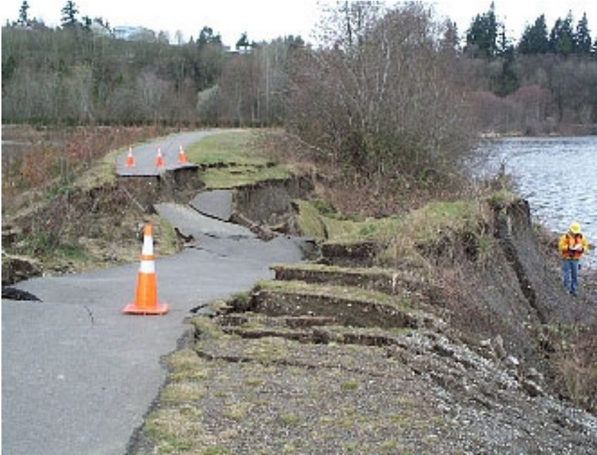
Figure 16–Site c, Figure13–East-to-west view of lateral spread of embankment at Capitol Interpretive Center. The length of the damage is approximately 75 feet (225 m) (Photo from Bray and others, 2001). (GPS location: N47.02396°, W122.90660°).
