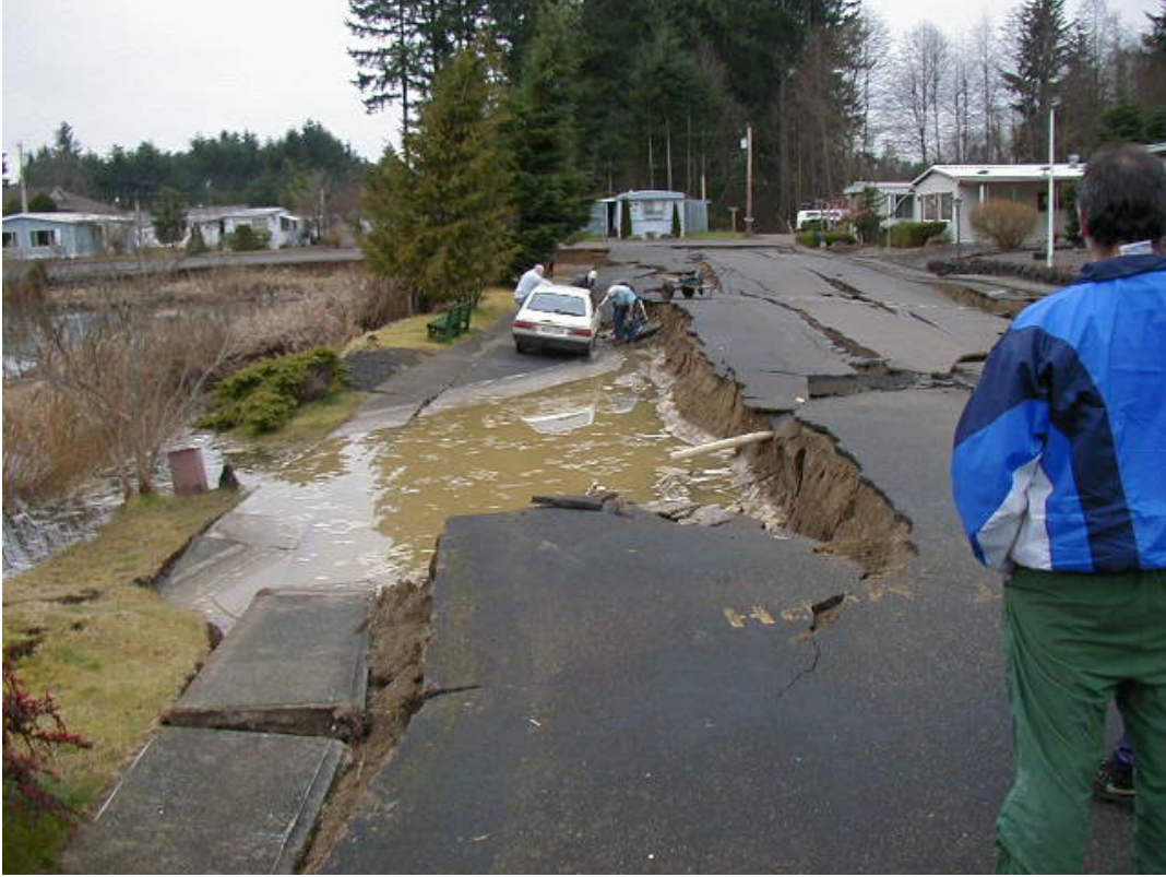
Figure 20—Close-up view of road failure at Sunset Lake, near Tumwater (Photo by Steven Kramer, University of Washington, Seattle).
