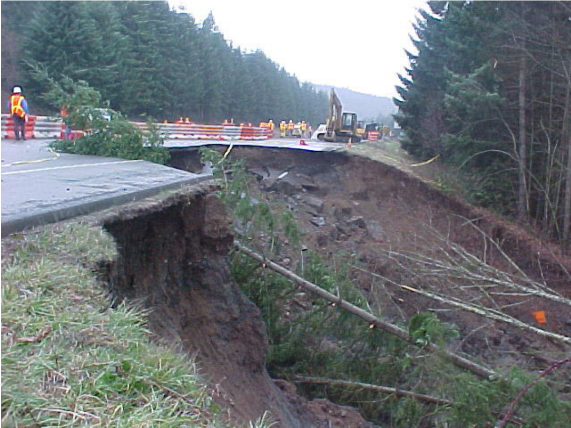
Figure 22—Close-up of U.S. Highway 101 landslide. The curved headscarp of the landslide is 24 m wide, and the total width of the landslide at the edge of the road is 35 m (Photo from Bray and others, 2001) (GPS location: N47.05834, W123.01365°).
