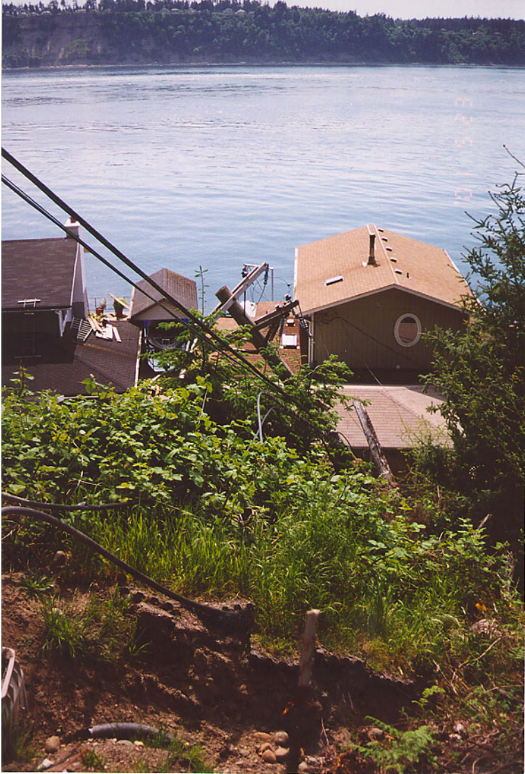
Figure 7—Looking toward Puget Sound from the Salmon Beach landslide. The landslide damaged electrical utility poles and electrical lines in the Salmon Beach community (Photo taken June, 2001 by Lynn Highland, USGS).
