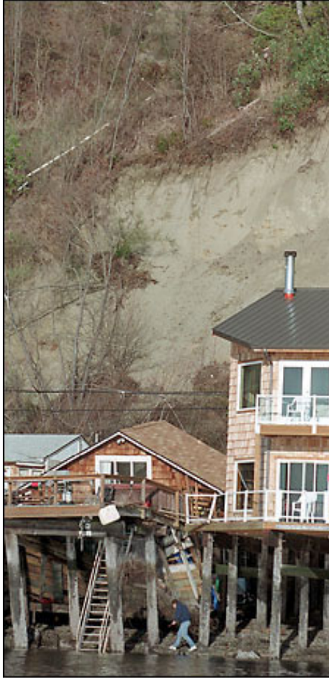
Figure 4—Close-up photo of one of the Salmon Beach houses damaged by a landslide, shortly after the Nisqually earthquake occurred (Photo courtesy of The Seattle Times).
