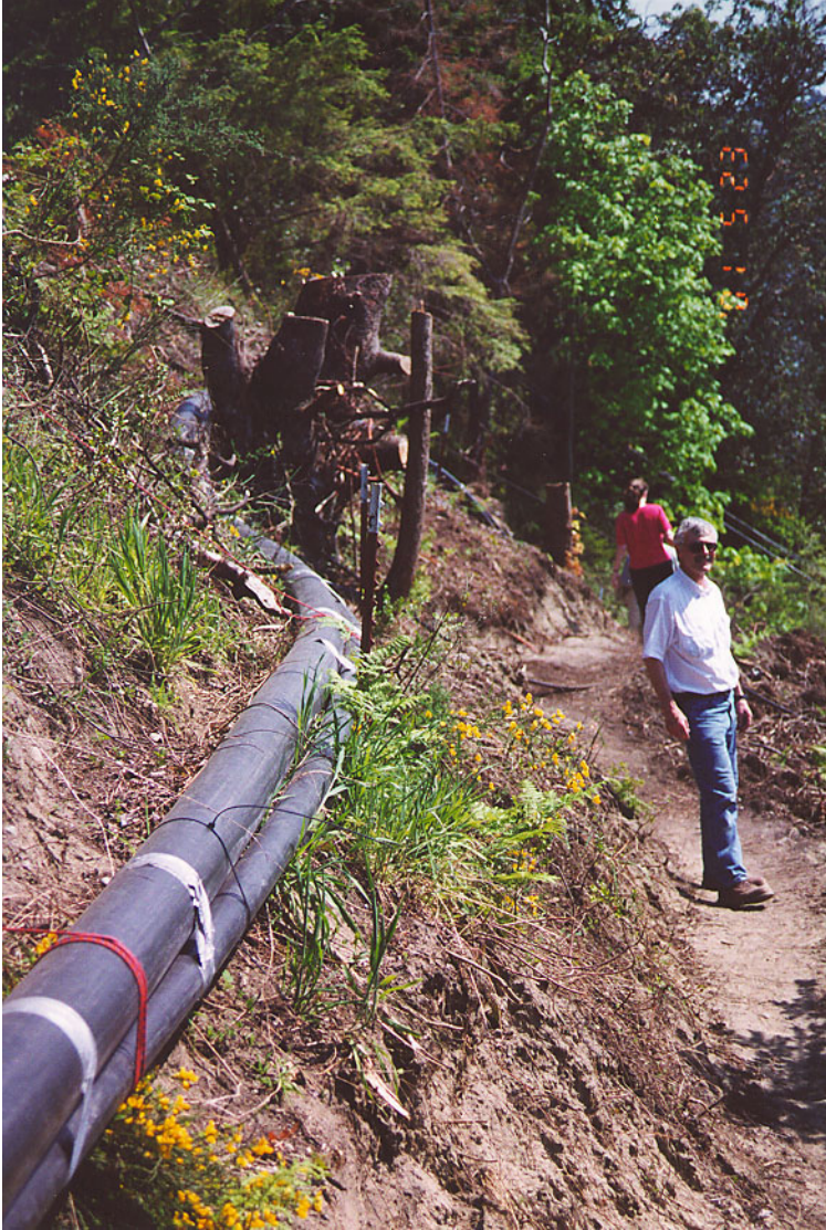
Figure 6–water and sewer line, temporarily relocated on top of landslide material, Salmon Beach landslide. Original sewer and water lines were damaged by the slide (Photo taken in June, 2001 by Lynn Highland, USGS).
