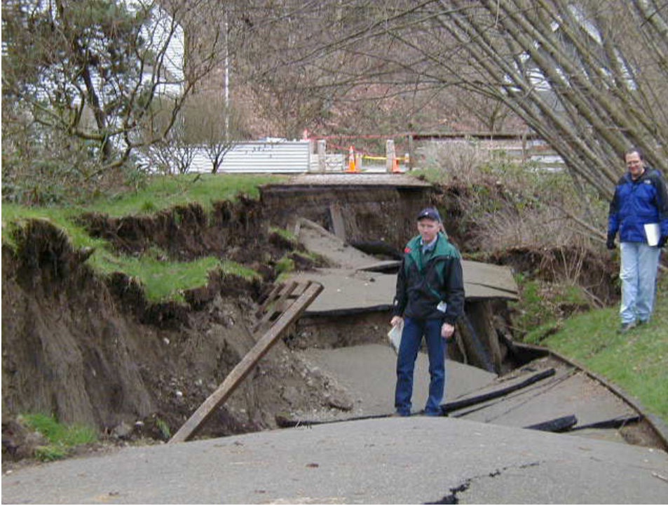
Figure 12–Capitol Lake, Olympia, landslide damage (Photo courtesy of WSDOT, February, 2001).
