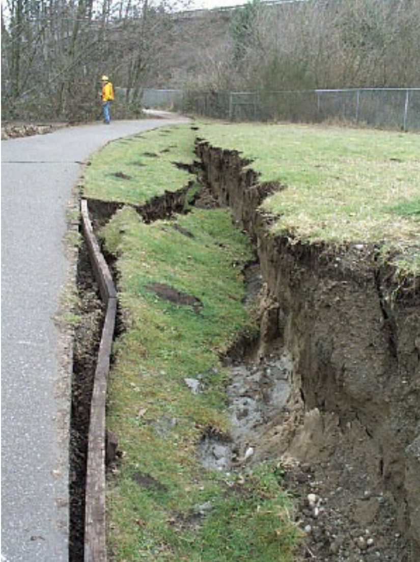
Figure 15–Site b, Figure13–Lateral spread of embankment at Capitol Interpretive Center (Photo from Bray and others, 2001). (GPS location: N47.04270°, W122.91090°).
