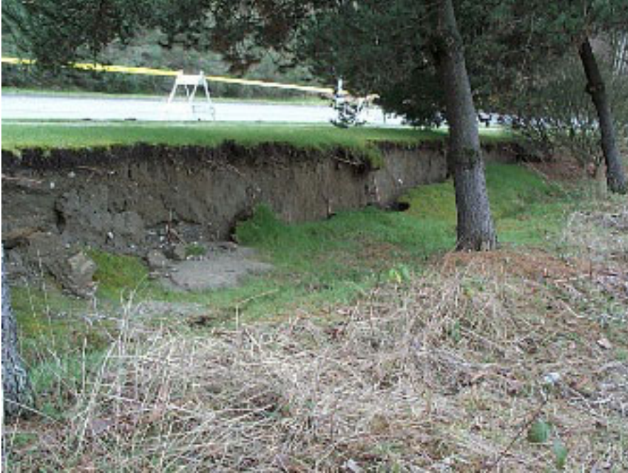
Figure14—Site a, Figure 13—Headscarp of lateral spread showing remains of sand boil (after heavy rain). The total length of the scarp is approximately 200 feet (60 m) with a maximum vertical drop of 3 feet (1 m) (Photo from Bray and others, 2001).
