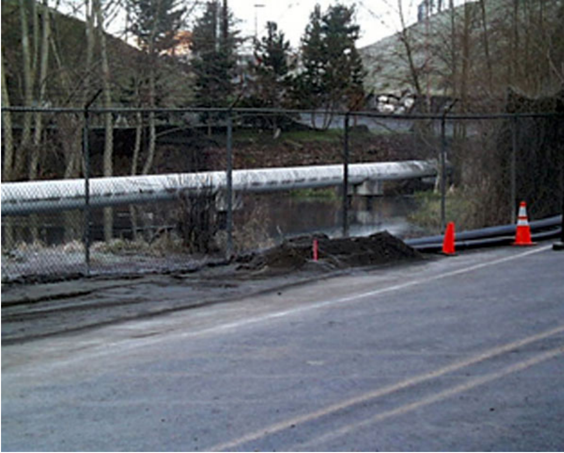
Figure 25–Chambers Road embankment failure and landslide. Sewer line repair using high-density polyethylene. Water-distribution line (undamaged) crosses adjacent to the bridge. Behind the water line on the far bank is a small landslide with several trees within sliding block (Photo by Bray and others, 2001) (GPS location: N47.1917°, W122.5733°).
