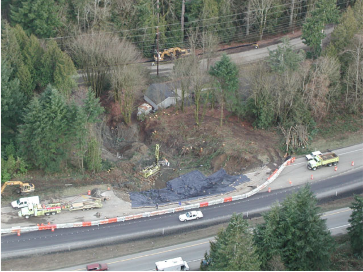
Figure 21–Landslide in U.S. Highway 101 road embankment near State Road (SR) 8 junction, northwest of Olympia. The earth embankment crosses a ravine that was carrying water at the time of the earthquake. The failed material moved down slope approximately 150 m and partially covered the road that parallels U.S. Highway 101 to the north (Photo from Bray and others, 2001) (GPS location: N47.05834°, W123.01365°).
